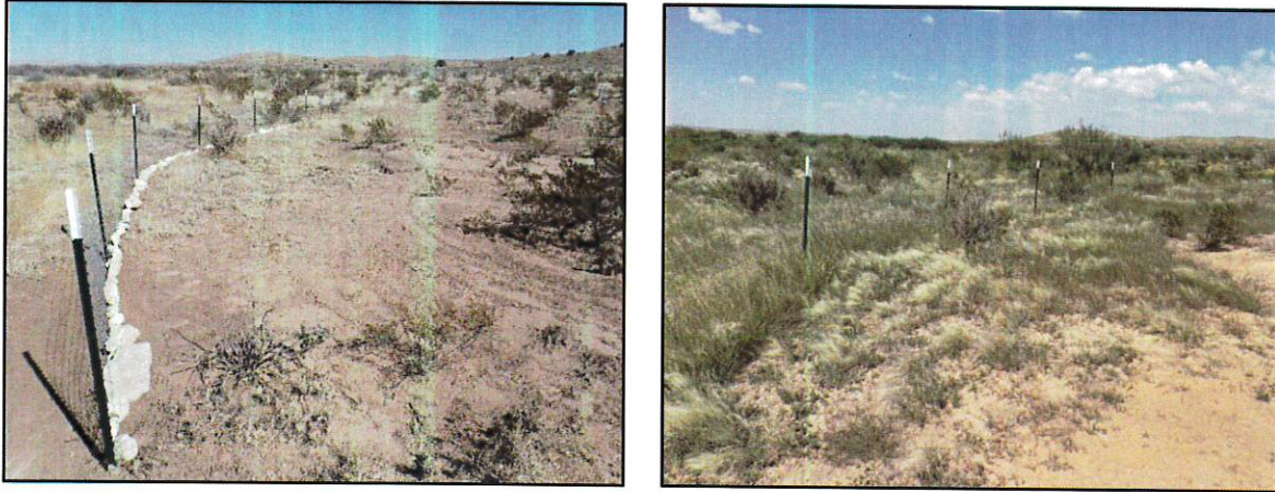
Figure 7. Before and After of Erosion Control Structures Used to Slow the Flow of Water and Catch Sediment.
